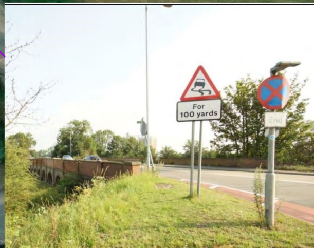
The south-west elevation has been repaired several times since due to road traffic accidents. About 30% of the south-western elevation brick-built parapet wall has been replaced during these repairs.
