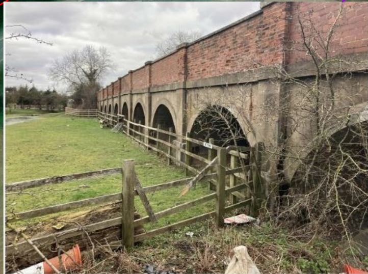
The potential impacts to the Causeway Arches were accepted by the Newark & Sherwood District Council Conservation Officer and the modern repair work from vehicle crashes on the western parapet were noted. It was advised that impacts should be restricted to the western side where possible.
