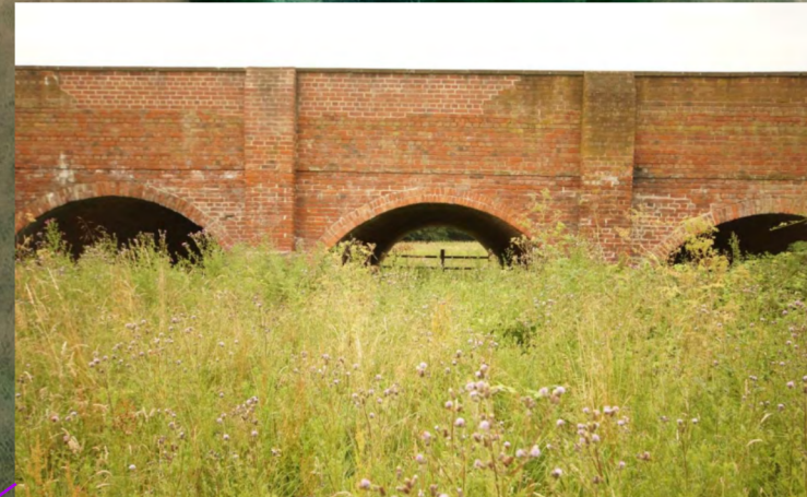
The north-east elevation has original brickwork. Three semi-circular arches have been repaired and replaced. Two central sections have been repaired with modern brickwork following a series of road traffic accidents.
