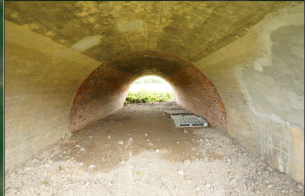
On the north-east elevation, internally, each archway leads to a barrel-vaulted passageway of original construction. On the south-west elevation, the arches were widened by approximately 4.25 meters in concrete construction.
