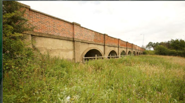
The south-west elevation was wholly rebuilt during the widening of the Great North Road in 1922. It is built of reinforced concrete with an upper brick-built parapet wall of 6 courses with coping stones.
